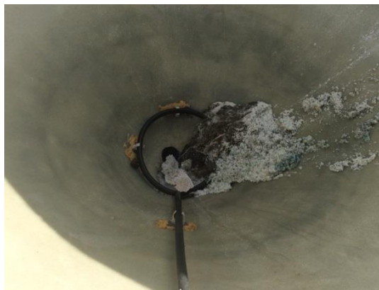
Empty salt hopper & dilution tank
